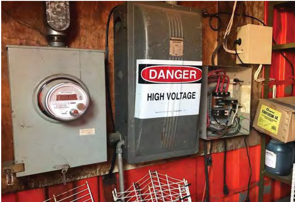
Figure 6: Electrical panels in workshop.
