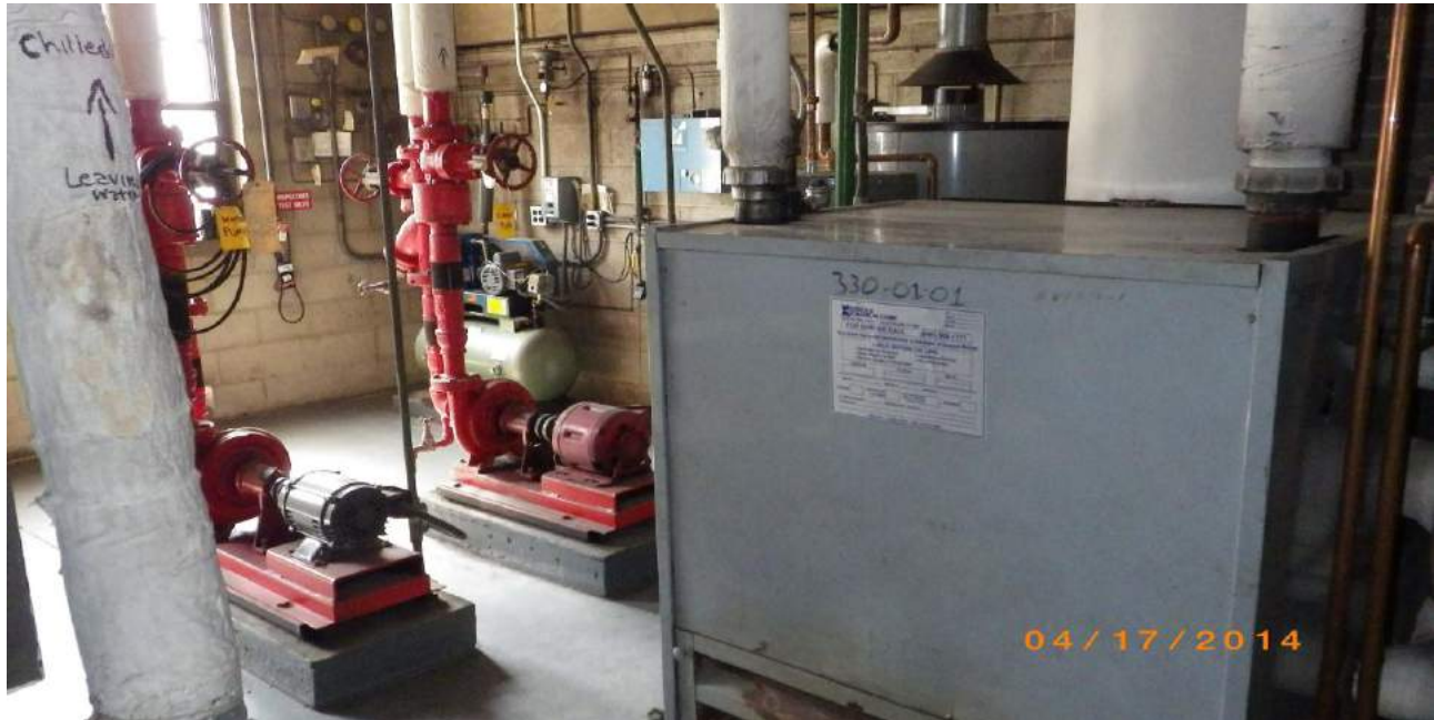
Photo 59: View of the boiler room located in the eastern area of the Third Avenue Transit Inc. building.
