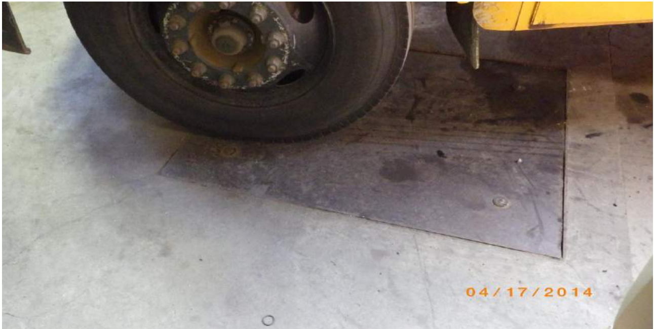
Photo 43: View of the oil/water separator.
