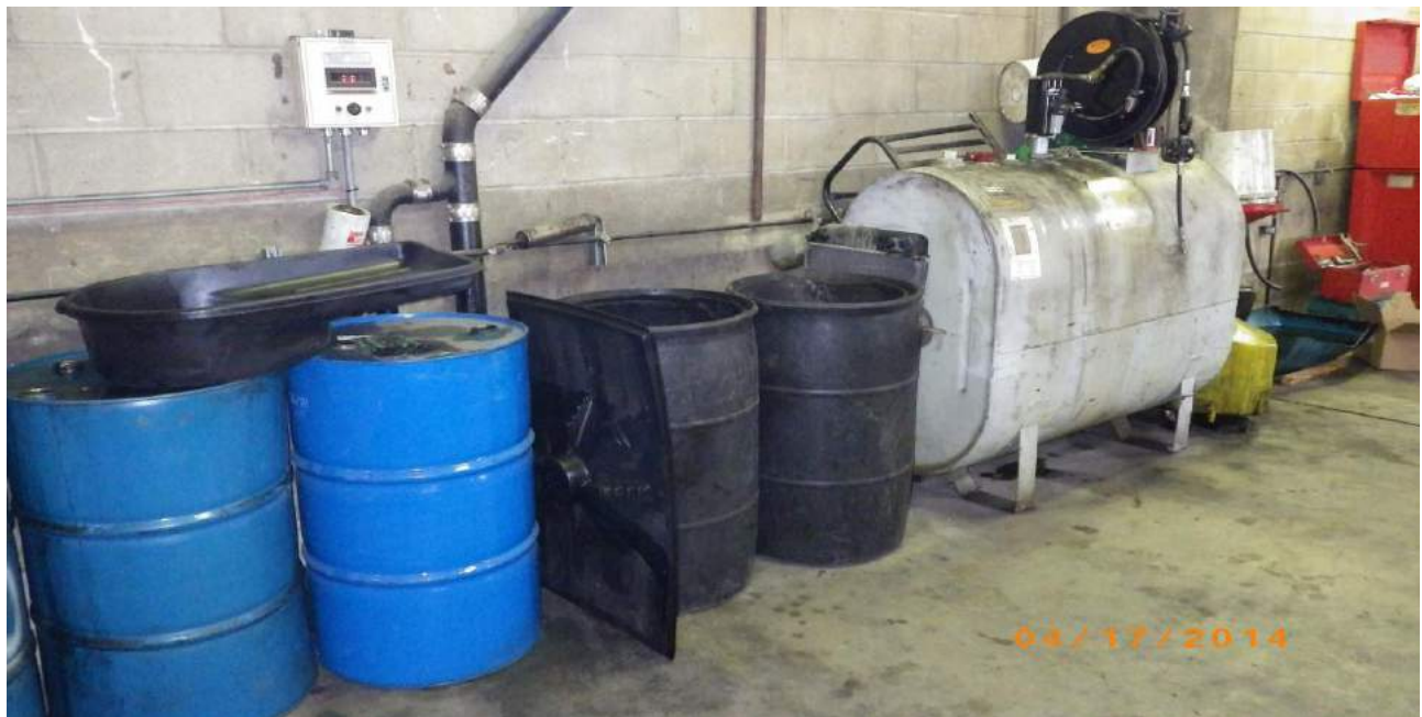
Photo 54: View of the 275-gallon hydraulic oil AST located within the Third Avenue Transit Inc. warehouse.
