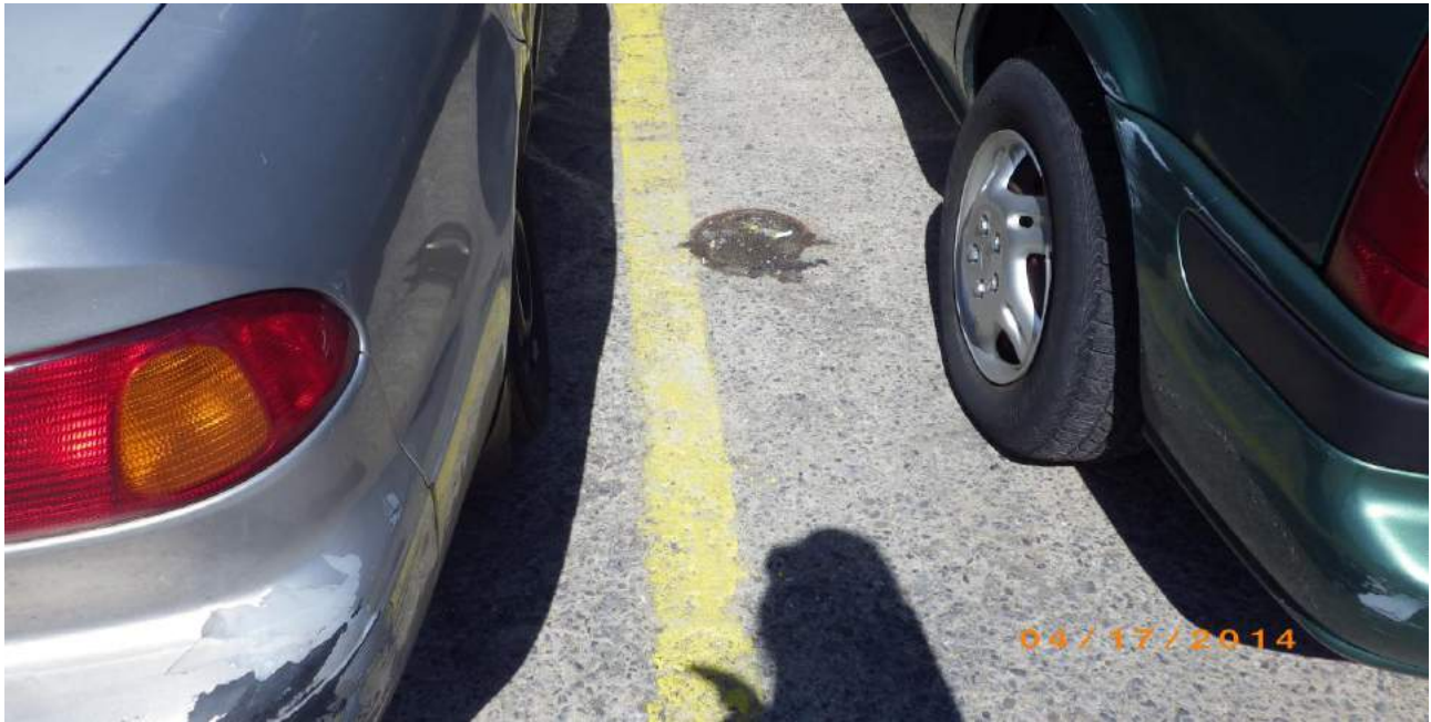
Photo 21: View of apparent historical fill port associated with the closed-in-place USTs along the eastern edge of the Site.
