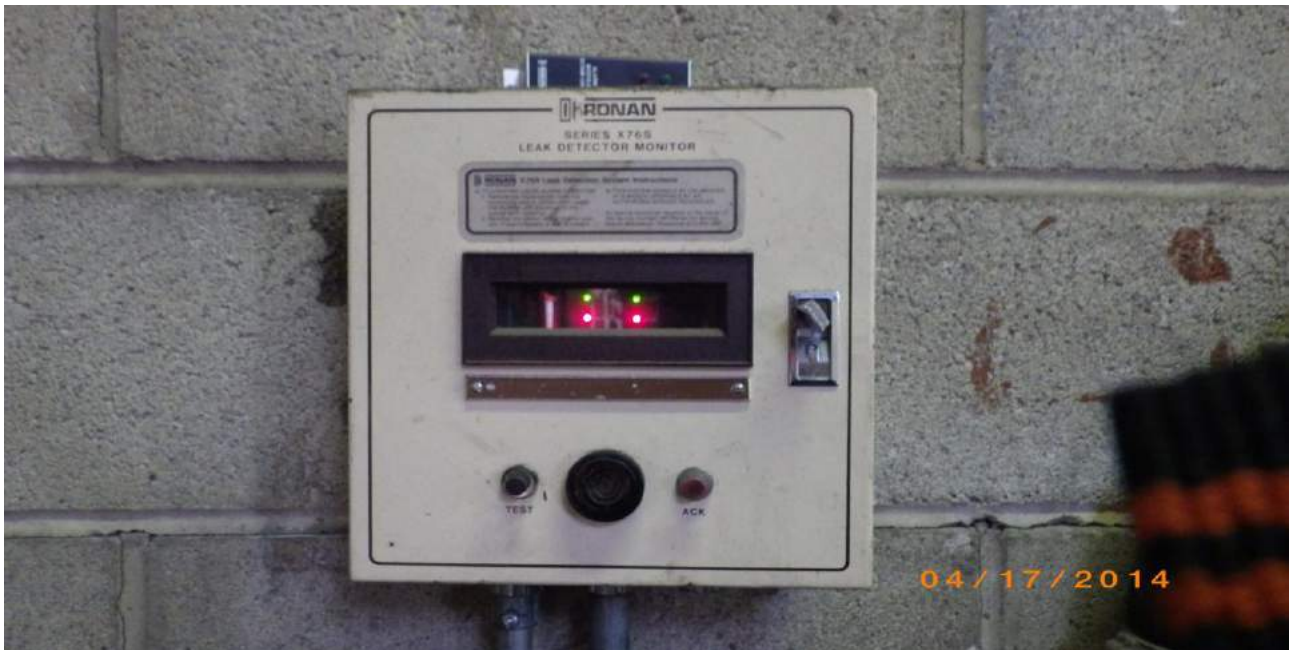
Photo 44: View of the apparent oil/water separator leak detector monitor.
