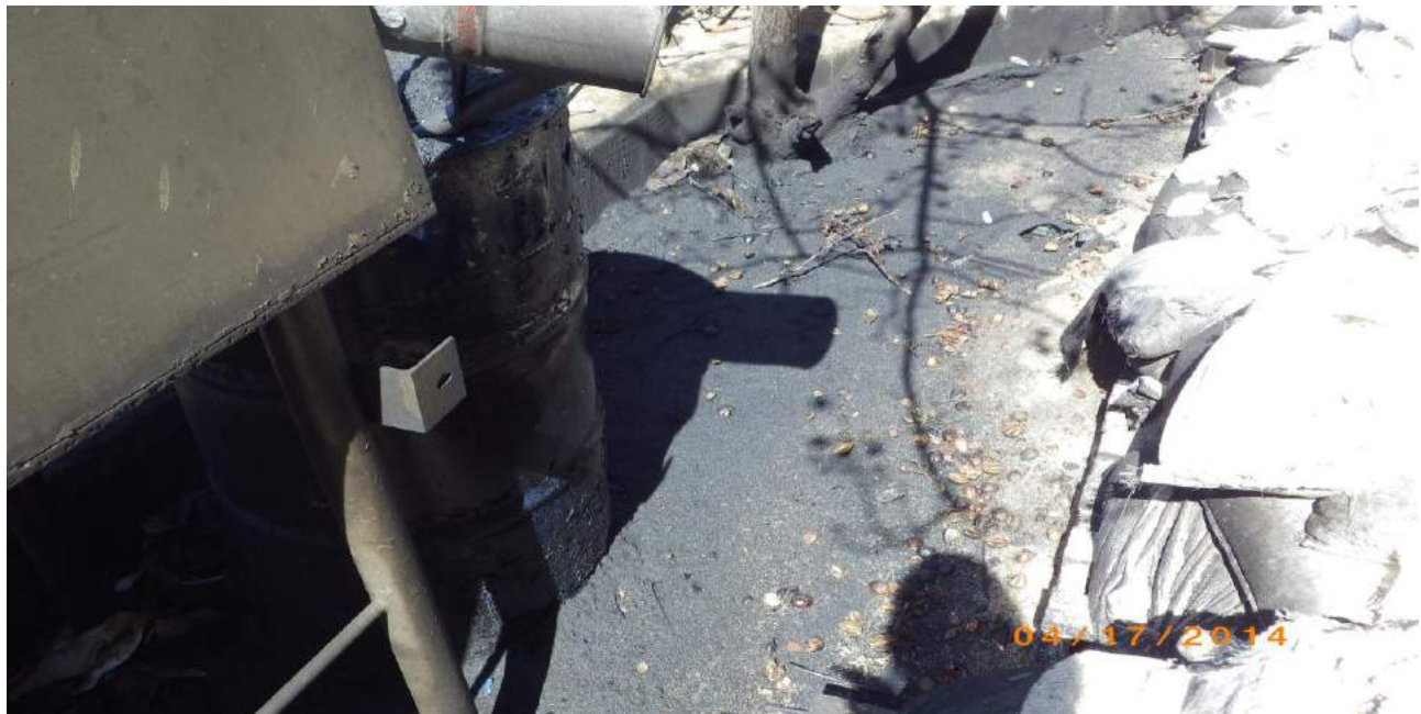
Photo 58: View of the corroded drum and soil staining area located immediately outside the Oz Moving & Storage warehouse, along the southwestern edge of the Site.
