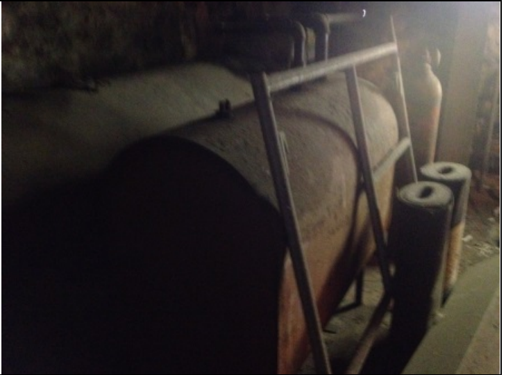
PHOTO 10: Looking at a second 275-gallon AST and behind that is another AST encased within concrete.
