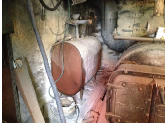
PHOTO 8: Looking at the oil tank associated with the oil fired hot air blower heating system.
